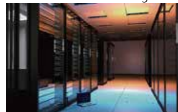
Data center thermal management
